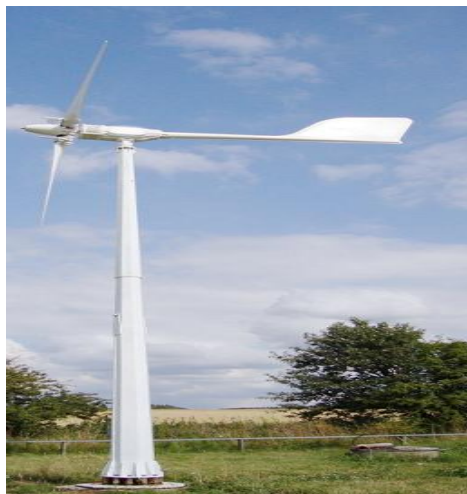
4.9 Kw wind turbine on an 8m pole
