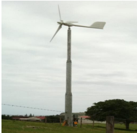
9.8Kw turbine – Princes Hwy Gerringong
