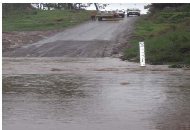
Dry River South – flooded, we turned back.
